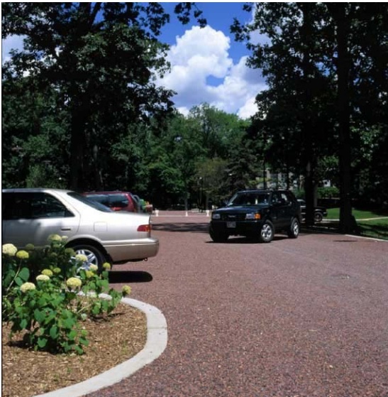
Grid pavers with gravel surface Dominican University, Illinois
